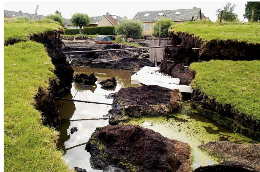
(Wilnis dyke failure, 26-08-2003)
